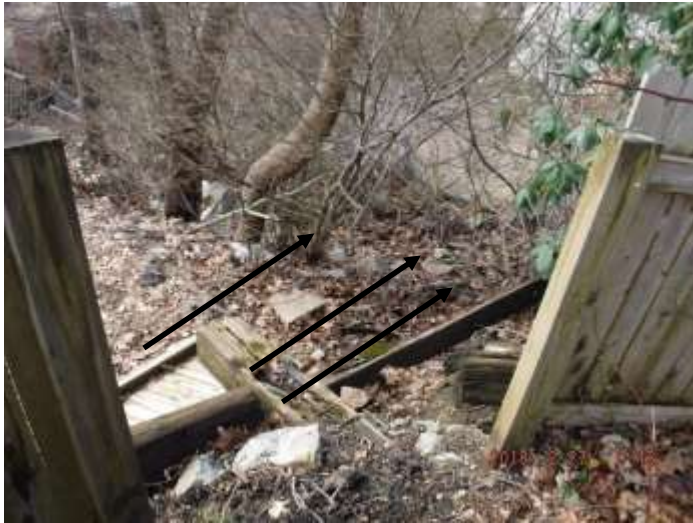
Figure 1 Steep drop off and missing/broken fencing. Fencing was loose, leaning, damaged and missing sections; safety hazards/dangerous.
