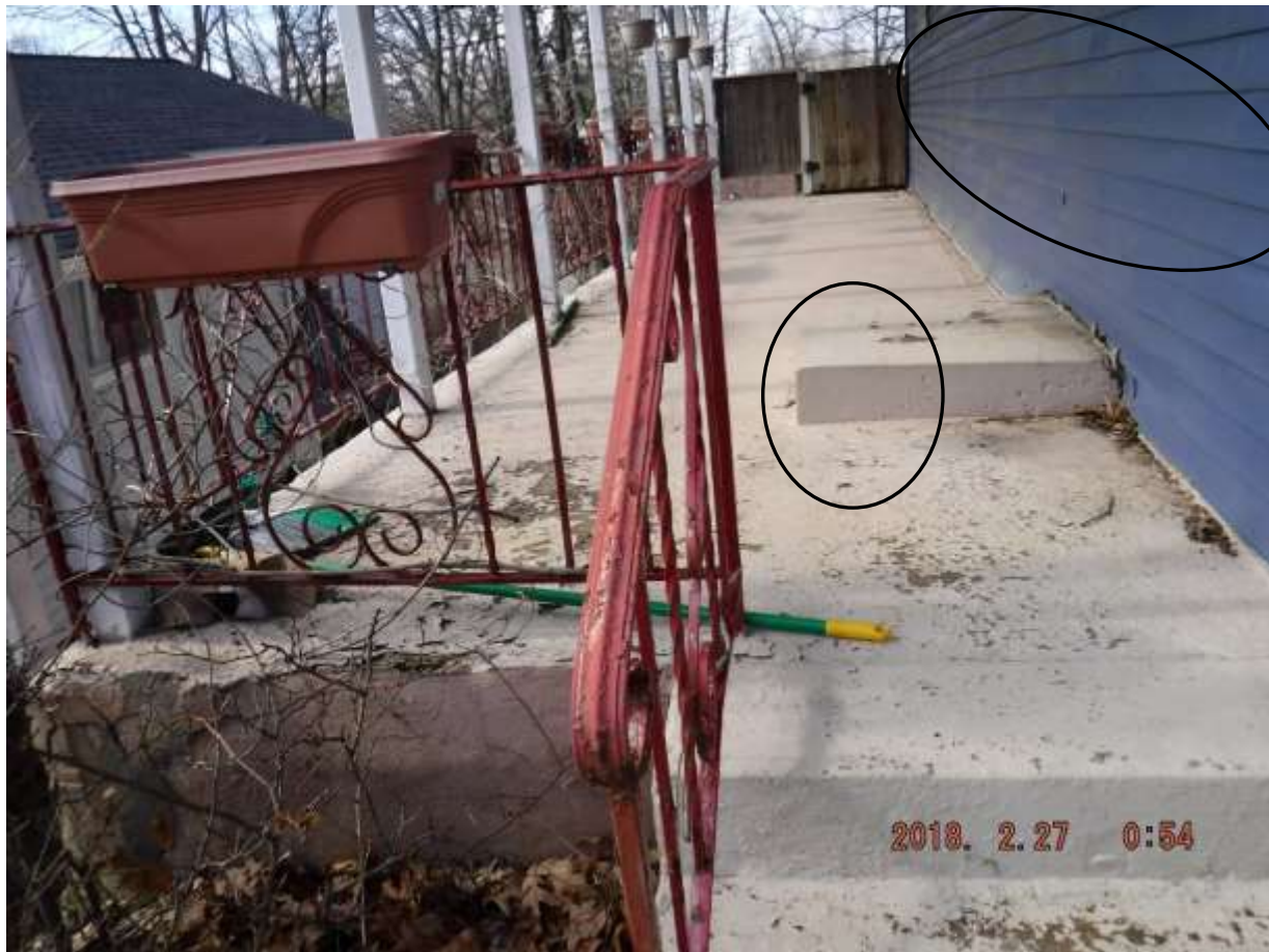
Figure 4 Slab from an enclosed door in living room. Siding had heat damage and wavy or buckled; further evaluate siding and causes before closing and contractual limitations.
