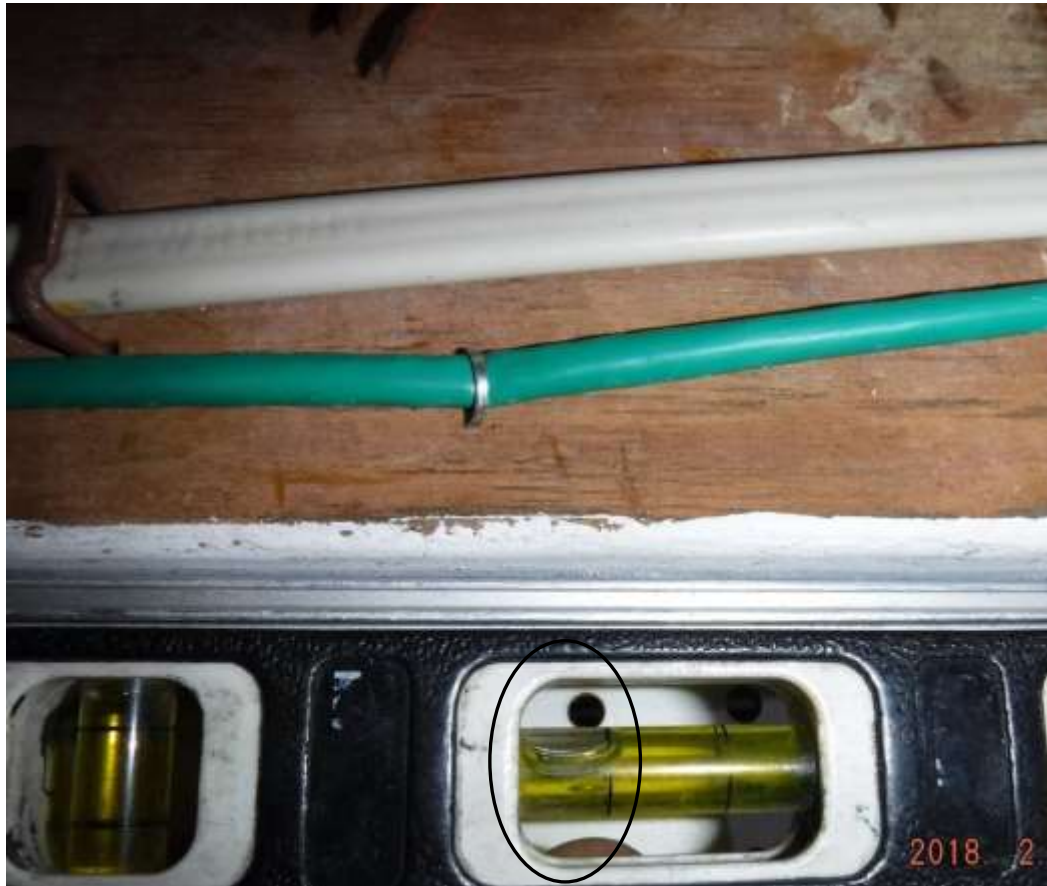
Figure 10 Broken/cracked built up beam on right basement; sloped flooring throughout the home.
