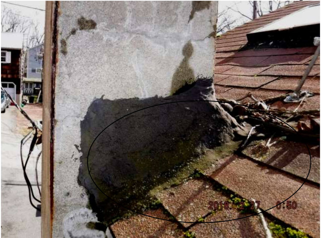
Figure 2 Roof was in poor condition; have evaluated for replacement, metal/proper flashings ( no tarring), skylights, ventilation, gutters.
