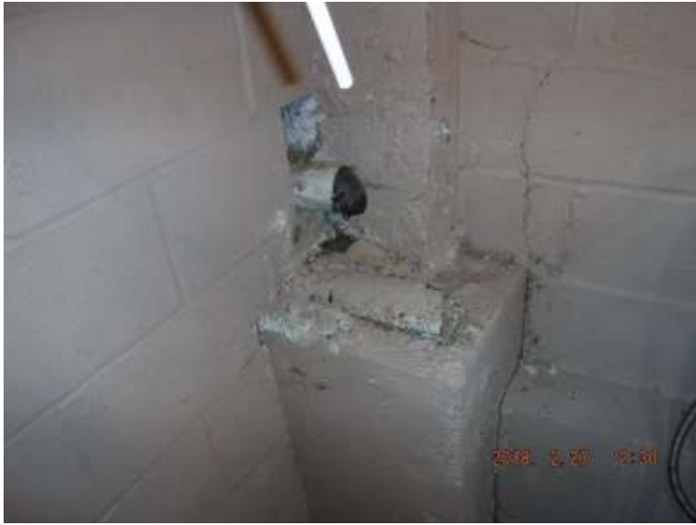
Figure 14 Further evaluate abandoned drains or piping in basement to rule out an abandoned septic on property.
