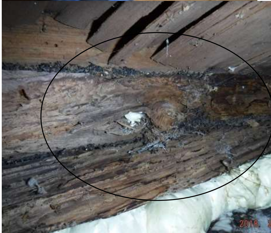
Figure 12 Moisture & carpenter ant damage to a beam on left side, mice droppings and carpenter ant frass.
