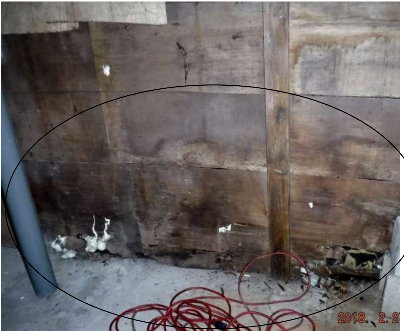
Figure 13 Water & dark staining, wood damage on wall under a damaged beam in basement.
