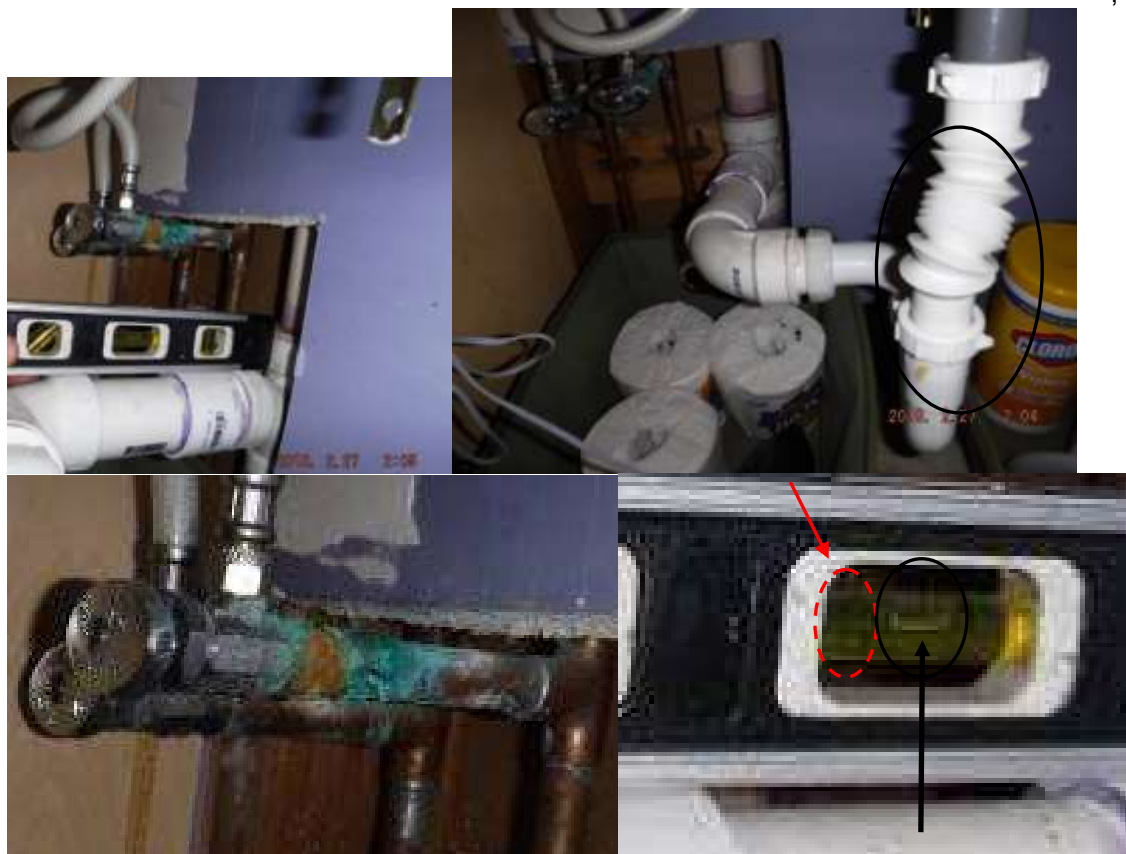
Figure 7 Example of corrosion, improperly pitched drain piping, flexible connector, etc.; improper drain installation. Recommend a licensed plumber evaluate all corrosion, drain installations and advise on repairs/corrections.
