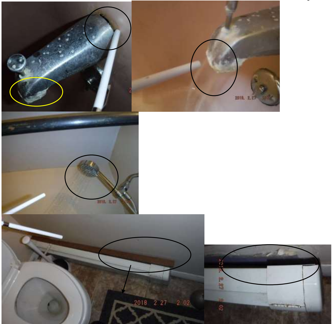
Figure 6 Example of loose baseboards in home; have an HVAC contractor evaluate/secure for safety.
