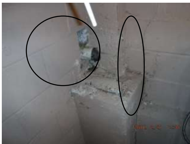
Figure 9 Abandoned piping or drains in basement; rule out an abandoned septic on property before closing. Example of foundation cracks and deepened basement or modified crawl space.
