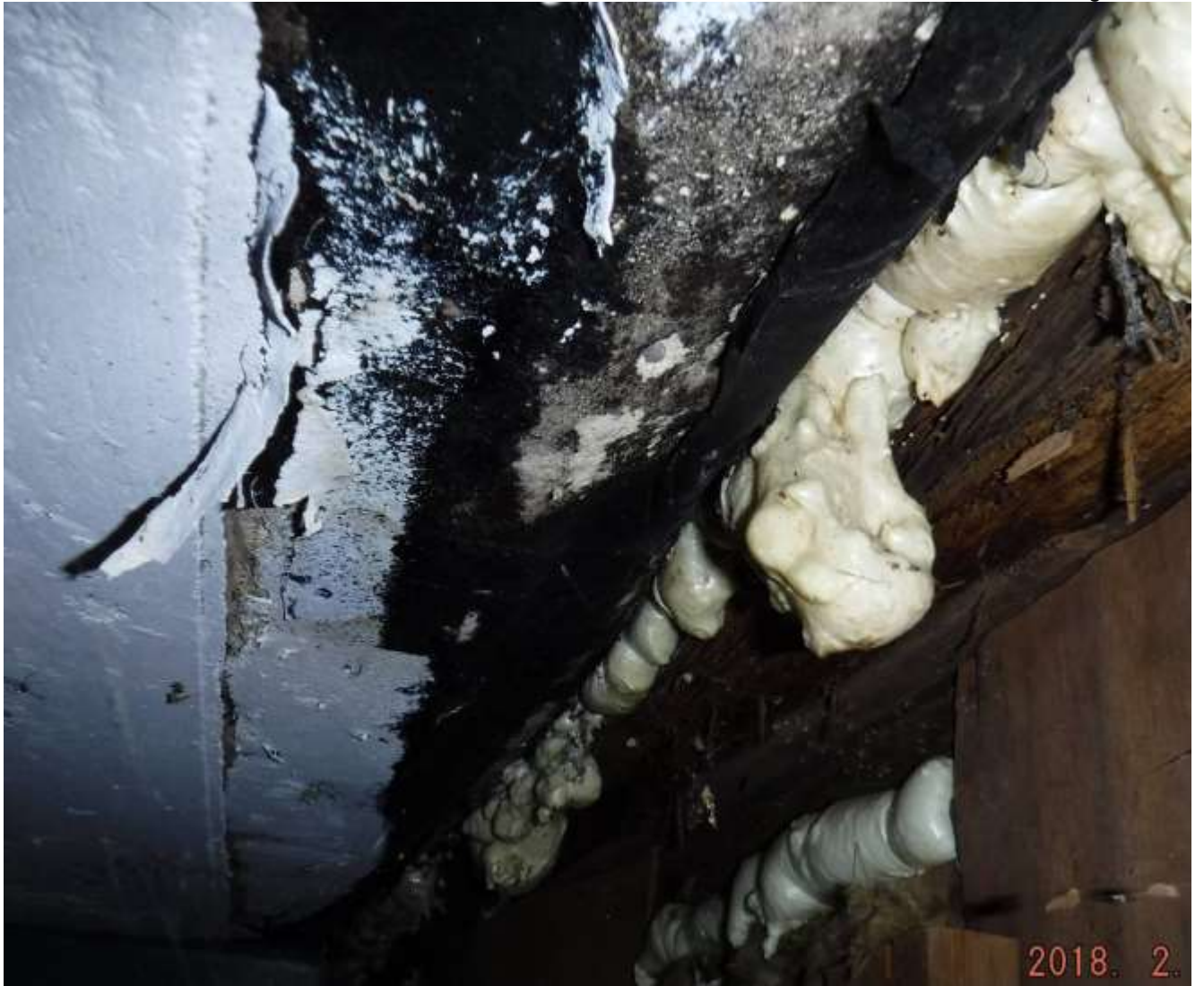
Figure 11 Example of damaged beam, rot and spray foam along the structure.
