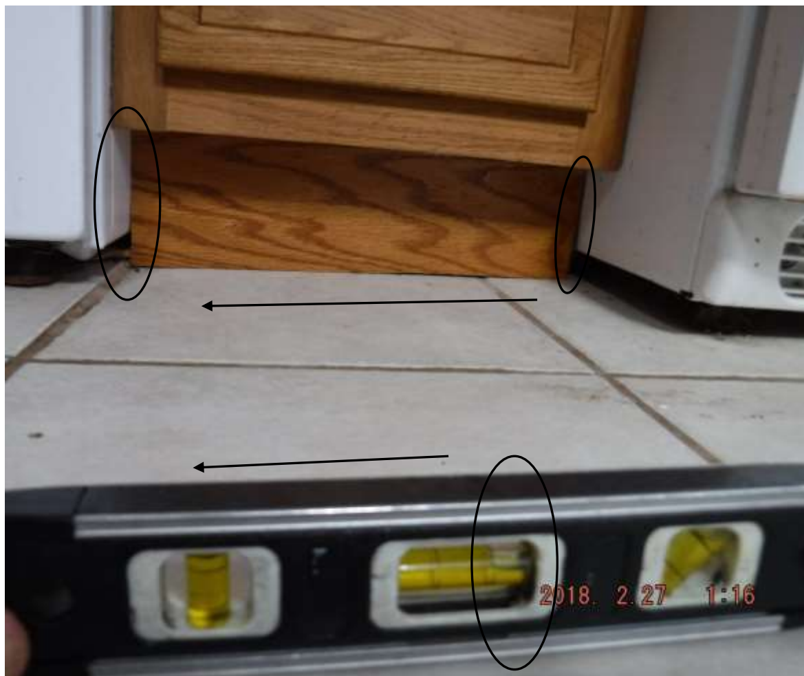
Figure 5 Example of sloped flooring and wedged base cabinet molding. See structural comments in basement and pg. 2 main concerns.
