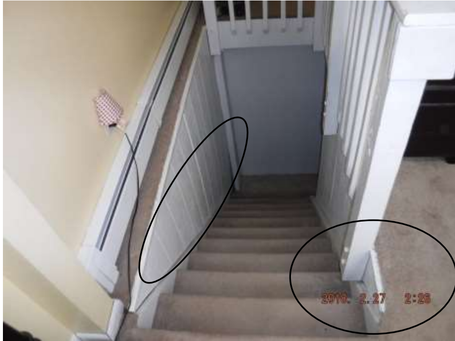
Figure 8 Railings should extend all the way across the steps and railing on steps for safety.
