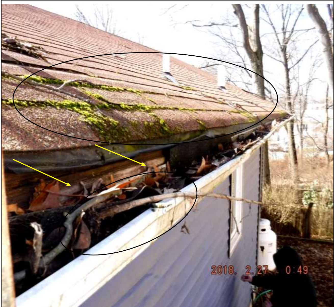
Figure 3 Water damaged/exposed wood, roof shingles old and poor condition. Recommend a roofer evaluate roof and advise on roof replacement, ventilation, gutters, skylight before closing & contractual limitations. Gutters, roof and exterior were in poor condition; see roofing, gutters, exterior/siding comments.
